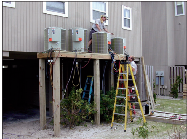
Elevated air conditioning compressors.
