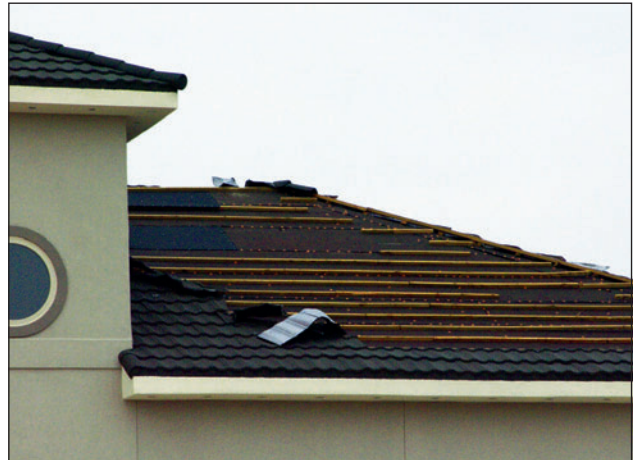
Figure 7. This residence had metal shingles that simulated the appearance of tile. The shingles typically blew off the battens, but some of the battens were also blown away.
