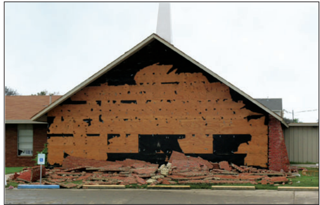
Figure 1. Failed brick veneer over plywood. Many of the ties are still attached to the substrate, but several of the tie fasteners pulled out of the substrate and the ties are embedded in the collapsed veneer. Estimated wind speed: 107 miles per hour (peak gust, Exposure C, at 33 feet).
