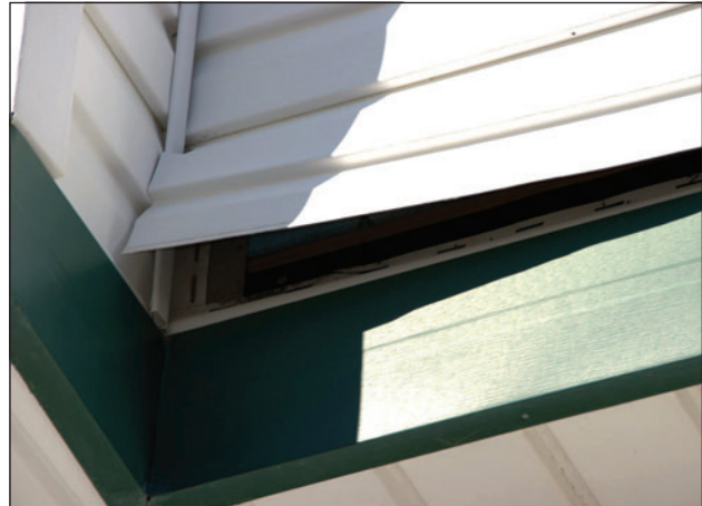
Figure 4. Utility trim was substituted for the starter strip and the bottom lock was cut off the siding. Siding was able to pull loose under wind pressure.
