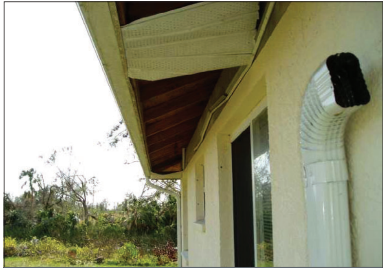
Figure 1. Missing soffit material.
