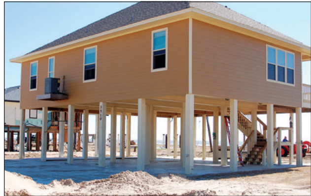
Figure 2. Breakaway walls beneath this building failed as intended under the flood forces of Hurricane Ike.
