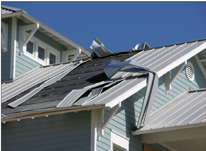
Figure 2. This architectural panel system has concealed clips. The panels unclipped from the clips. The first row of clips (just above the red line) was several inches from the end of the panels. The first row of clips should have been closer to the eave.
