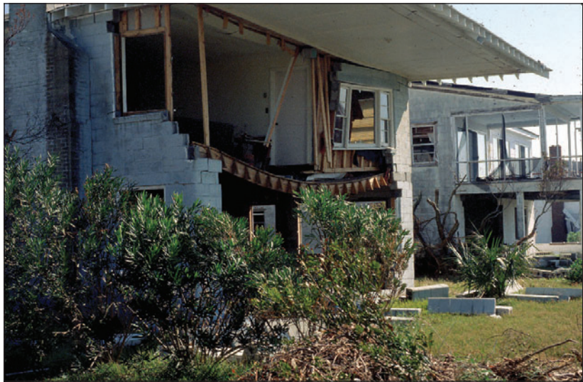
Figure 1. Storm-damaged homes need repairs, but also provide opportunities for renovation, additions, and retrofitting. Review substantial damage and substantial improvement regulations before undertaking any work.
