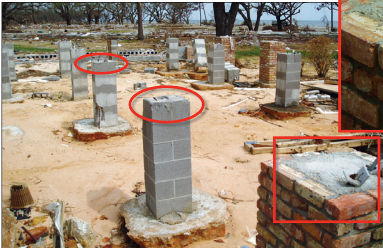
Figure 3. Failure of pier-to-beam connections due to wave and flood forces acting on the elevated building (Long Beach, Mississippi)
