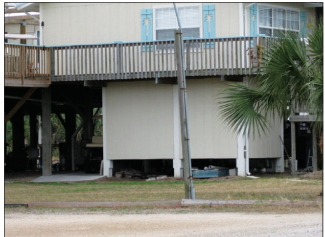
Figure 6. Example of an enclosure that does not extend to grade. This type of enclosure presents special construction and flood insurance issues. Contractors should proceed with caution when an owner requests such an enclosure.
