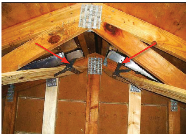
Figure 12. Metal plugs (red arrows) in gable rake vents.
