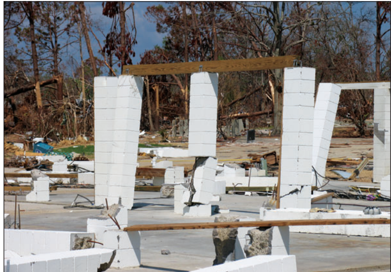
Figure 2. Pier breakage (Long Beach, Mississippi)
