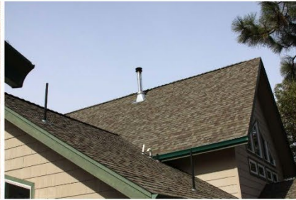
Keep over hanging tree limbs pruned at least 10 feet away from chimneys and stove pipes. Use fire-resistant building materials.
